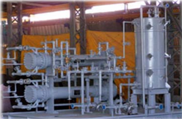
Aux. Skid packaging -Cooling water console Client - Dresser rand End User- Inelectra- Colombia
